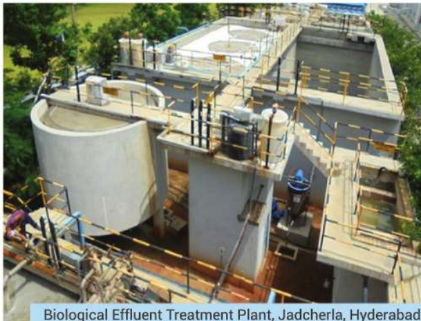
Biological Effluent Treatment Plant, Jadcherla, Hyderabad
